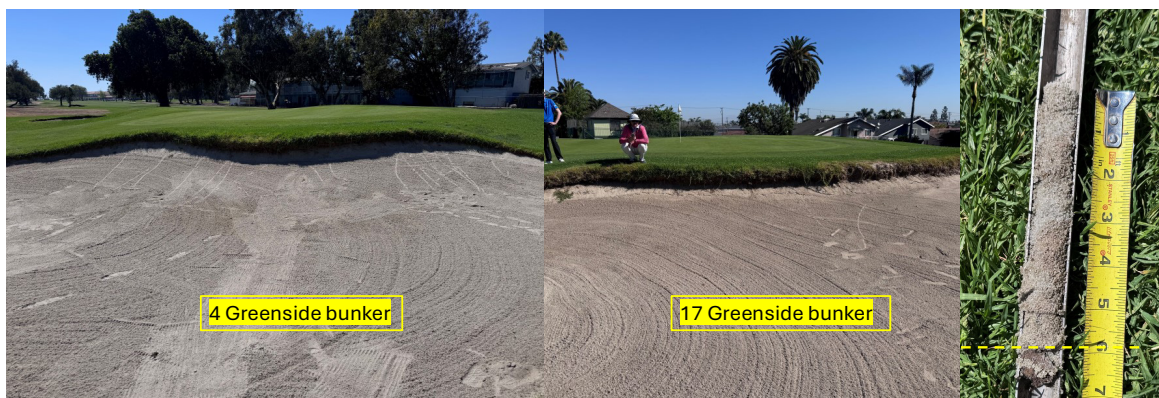
The bunker lips are likely 2 to 3 feet higher than their original elevation. Sand depth was measured at approximately 6 inches (right).
