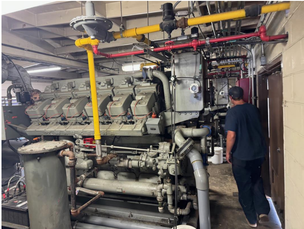
Hamilton Pump Station (2024)
