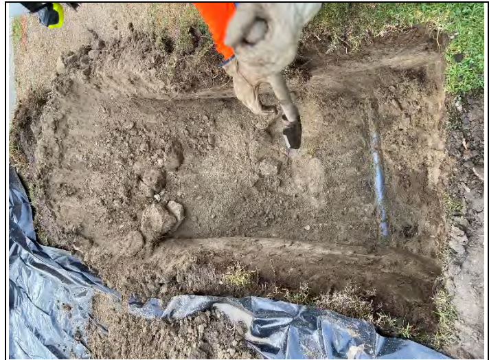
Electric utility pipe encountered at TP-3 (looking south).
