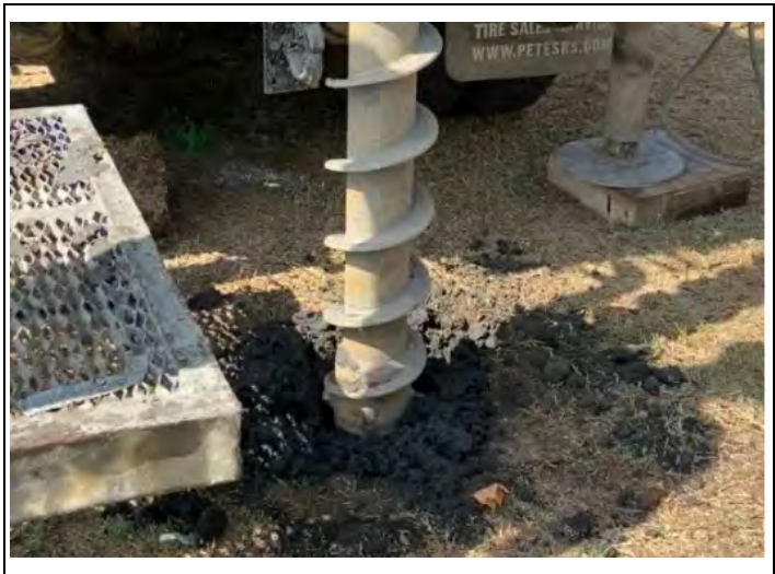
Waste encountered at HSA-4 (looking northwest).
