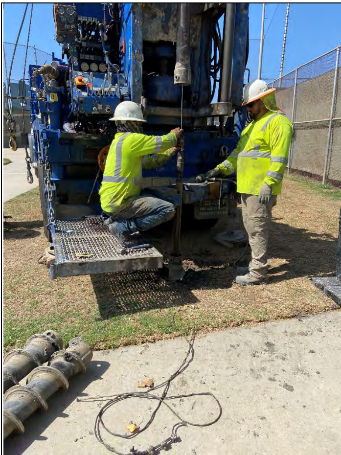
Damage to the wire connecting the sampling barrel assembly to the lead auger at HSA-4; ABC fixing the wire (looking west).
