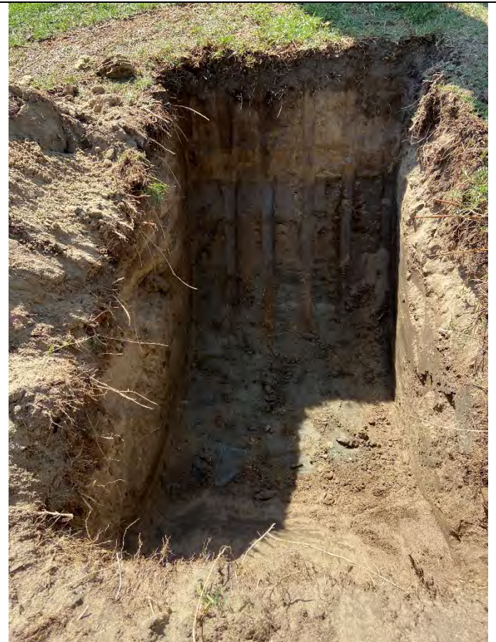
Pothole 35 ft east of excavated trench at TP-5 and observation of waste (looking west).
