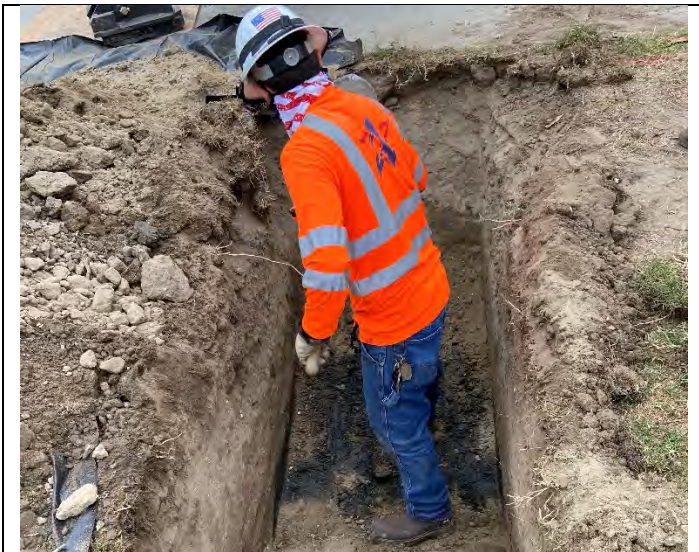
Waste encountered at TP-3, waste continues underneath the concrete slab (looking east)
