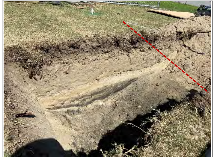
Waste encountered at TP-2 and the lateral limit of waste (looking northeast).
