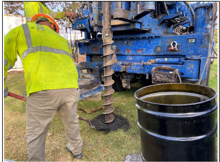
Waste encountered at HSA-5 (looking northwest).
