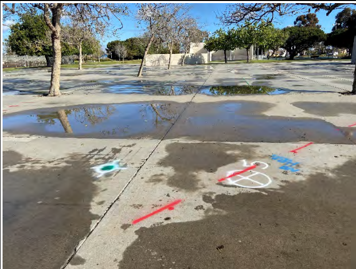
Electrical utility markings at existing HSA-5A and the new HSA-5A location (looking north)
