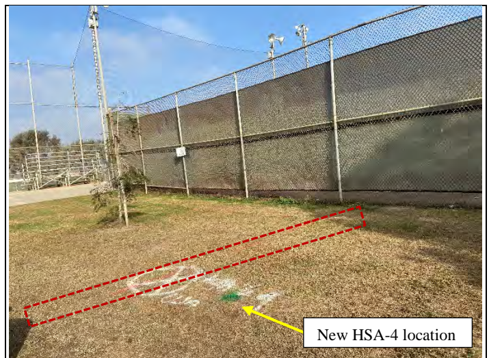
Utility markings at existing HSA-4 location and the new HSA-4 location (looking northwest)
