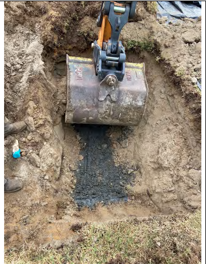
Waste encountered at TP-4 (looking east).
