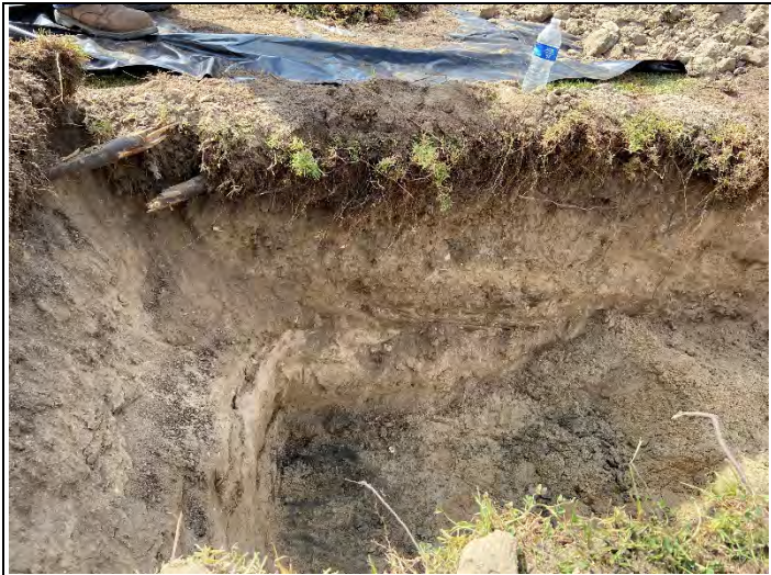
Waste observed to continue underneath the concrete slab at TP-4 (looking south).
