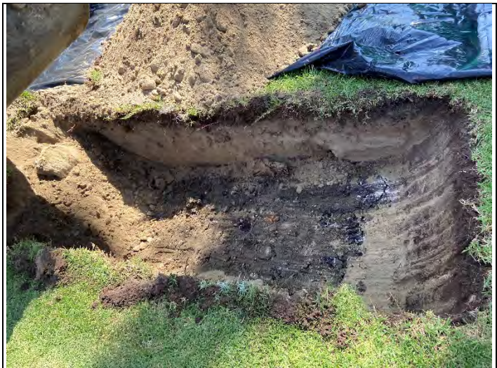
Waste encountered at TP-5 (looking south).
