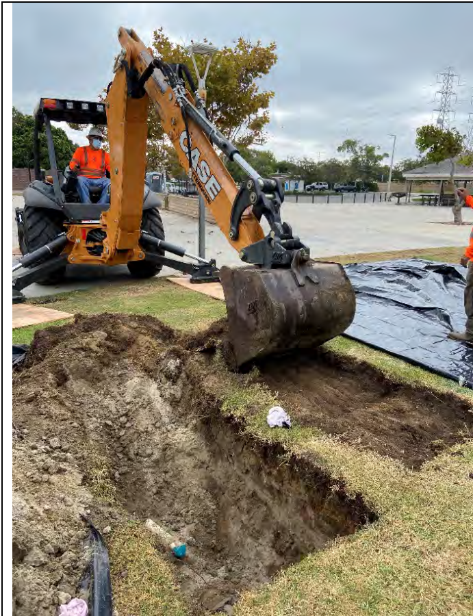
Excavation of second trench adjacent to the first trench at TP-4 (looking southeast).
