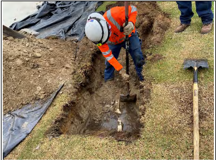
Damaged irrigation pipe at TP-4 (looking northeast).
